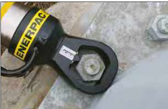
◀ Heavily corroded and weathered nuts are quickly split and removed using a NS-Series Nut Splitter.
